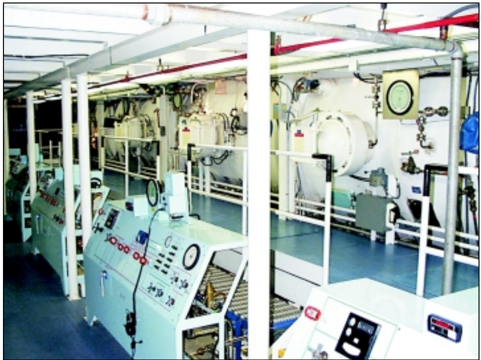
Figure 15-5. NEDU's Ocean Simulation Facility Saturation Diving Chamber Complex.
